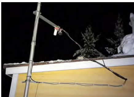
Above: Temperature and snow depth sensors installed above a roof.
